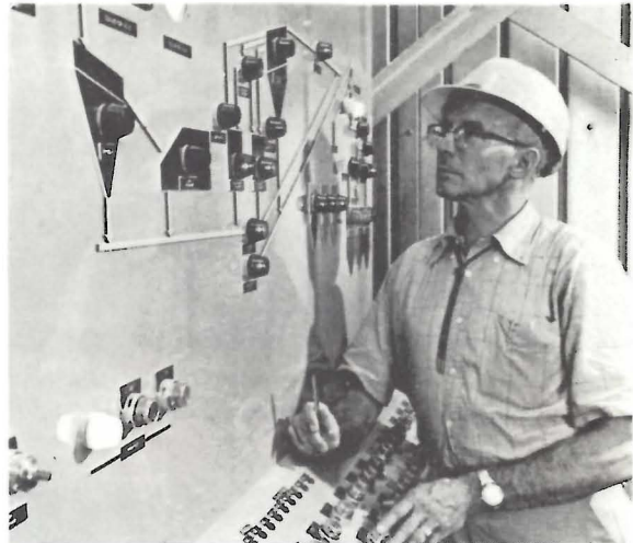
Photo 84. TANCO Mill, Main Control Panel, Bernic Lake (MED).
