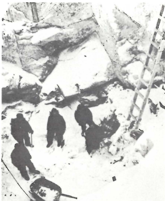
Photo 54. Collaring the EL Shaft, Sherritt Gordon Mines Limited, Lynn Lake Area (ca. 1948) (SGM).
