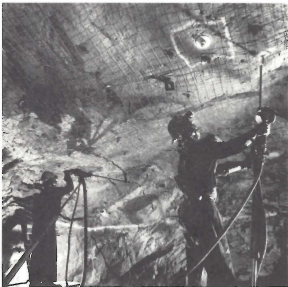
Photo 70. Roof Bolting. Photo illustrates the bolt-and-screen method of roof support. The miner at the right is roof bolting. The miner at the left is drilling the breast (INCO).
