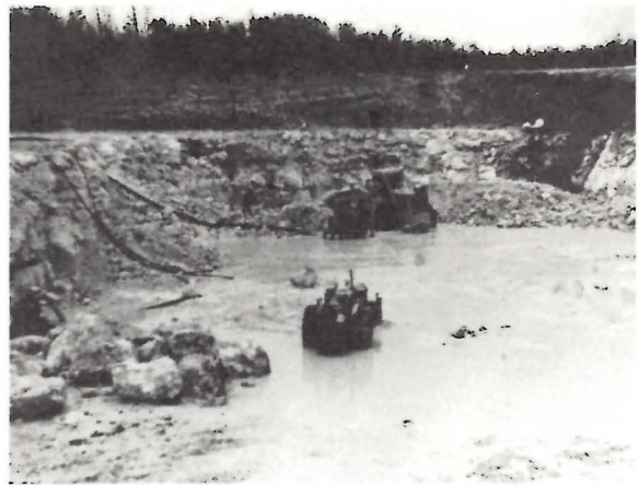
Photo 24. Mucking the Blast and Pumping Spring Run-Off. A time of flooding conditions in Southern Manitoba (MRD).
