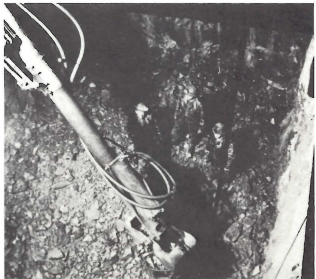
Photo 5. Drilling the Round — After all the holes have been drilled, they are loaded with explosives and blasted, breaking the rock and deepening the shaft (MRD).
