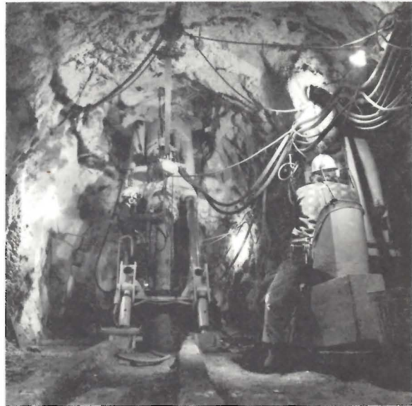
Photo 72. Raise Boring Machine at an Inco Metals Company Mine, Thompson Area. The raise is bored to its full size to provide access from one level to another (INCO).
